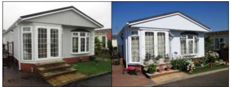
Before and After park home insulation - funded through the first phase of Local Authority Delivery funding (Green Jump Surrey), delivered by Action Surrey.
